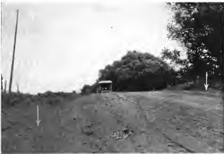
This is not a hill but a sharp cross ridge that has all the effect of a two-way grade. It will be noticed in the left foreground that a lot of labor has been expended without definite results. The same amount of work would have cut off the cross ridge, with consequent improved going in both directions.
